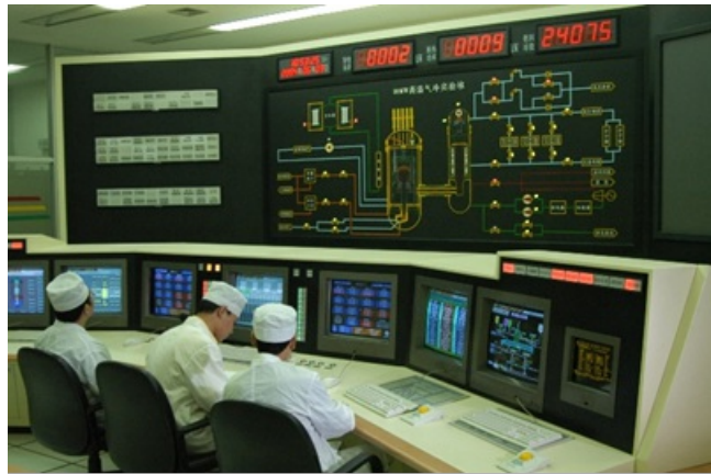
Figure 4. HTR-10 control room
