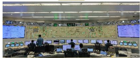
HTR-PM Main Control Room
