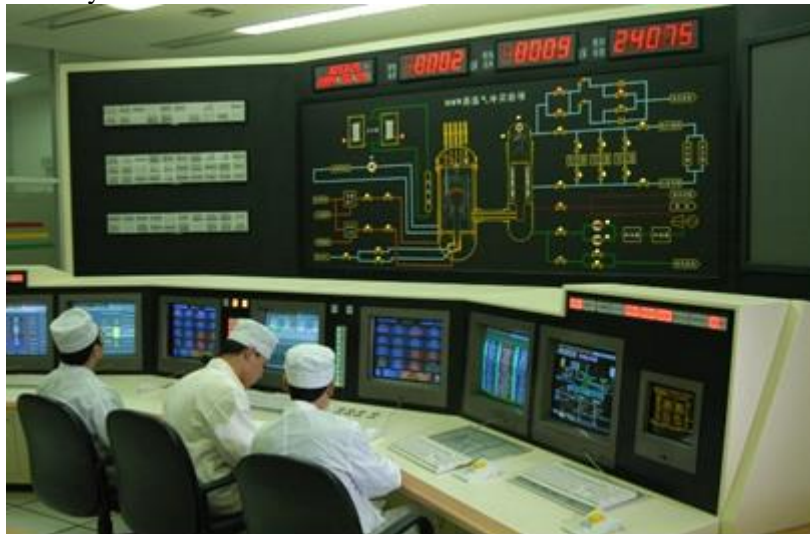
HTR-10 Control room
