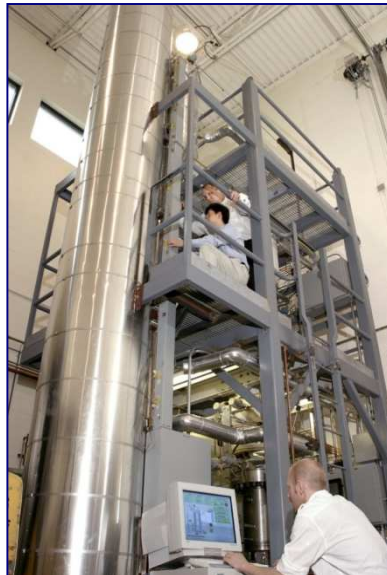
Figure 5. NuScale Integral System Test Facility at OSU.
